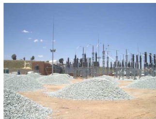
Meadow Substation, Nov 2003 132/11kV, 2x40MVA
